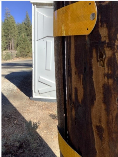
Exposed ground wire at 4 feet on pole BV11050 BV11050
